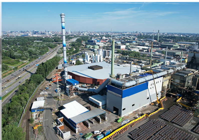
First RDE expansion stage at the Hamburg site
